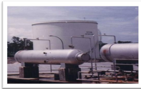
Crude Oil Tank PT. Petrochina Sorong 2002
