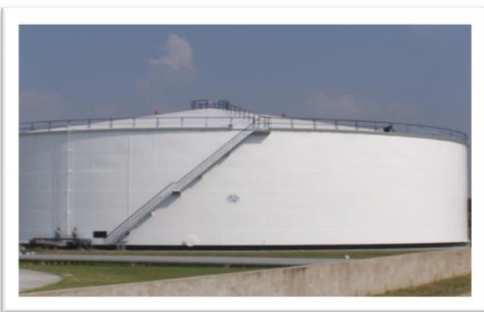
BBM Storage Tank Depot Plumpang PT. Pertamina UMS III 2006
