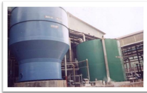
Buffer Tank PT. Indah Kiat Pup & Paper - Perawang 2003
