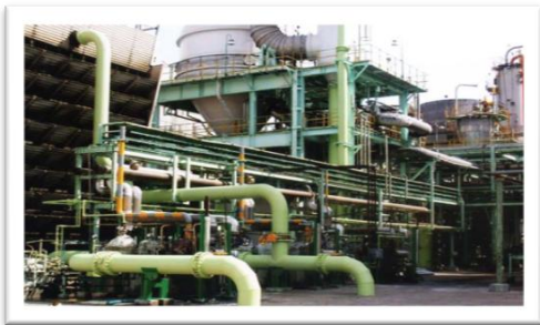
Plant Urea PT. PUSRI - Palembang 2004 - 2006
