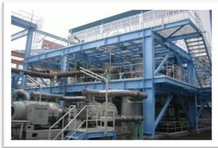
Structure Pipe Rack PT. Magma Nusantara Ltd 2009
