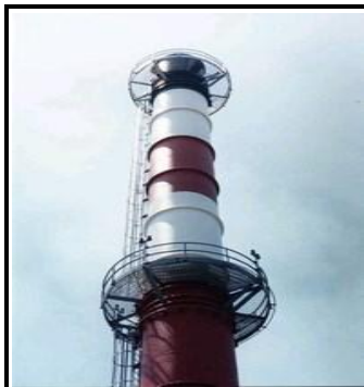
PT. Indonesia power UBP Semarang - PLTU 1&2 2004, 2008
