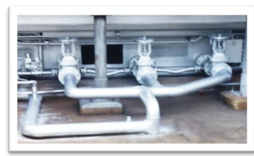
Exhaust Plenum Drain Pipe PT. Indonesia Power UBP Semarang 2004
