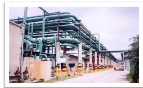
Water line Pipe PT. Indah Kiat Perawang 2003
