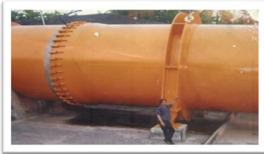
Pipa Pesat PT. Indonesia power UBP Saguling 2008
