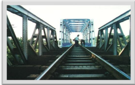
Railway Bridge PT. Perumka - 1992 Epoxy (75 micron) - Polyurethane (75 micron) Simacover EP Unicoat - Simathane Gloss
