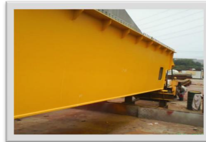
Jembatan Pela PU Bina Marga - 2007 Epoxy (75 micron) - Polyurethane (75 micron) Simacover EP Unicoat - Simathane Gloss
