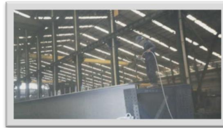
Railway Bridge PT. Bukaka Teknik Utama - 1993 Epoxy (75 micron) - Polyurethane (75 micron) Simacover EP Unicoat - Simathane Gloss
