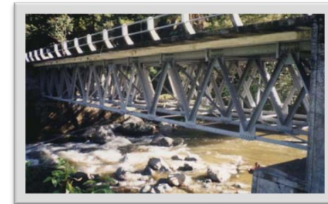
Jembatan Duku 2 PU Bina Marga - 1999 1999 Epoxy (75 micron) - Polyurethane (75 micron) Simacover EP Unicoat - Simathane Gloss
