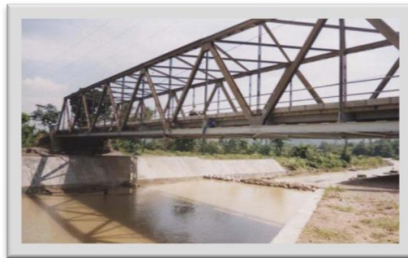
Jembatan Ciancur - Ciri PU Bina Marga - 2004 Epoxy (75 micron) - Polyurethane (75 micron) Simacover EP Unicoat - Simathane Gloss
