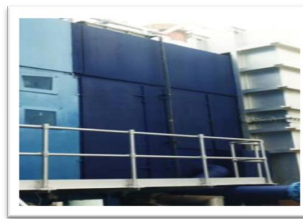
Generator Compartment PT. Indonesia Power UBP Semarang 2004
