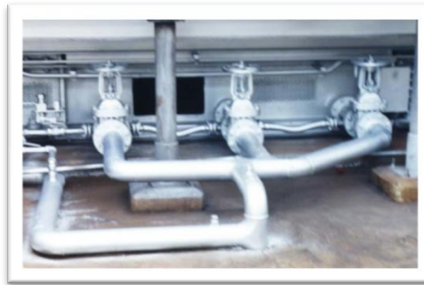
Exhaust Plenum PT. Indonesia Power UBP Semarang 2004
